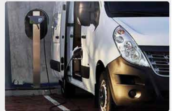
EV Charging Stations
