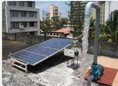
Solar Water Pumping for Institutions
