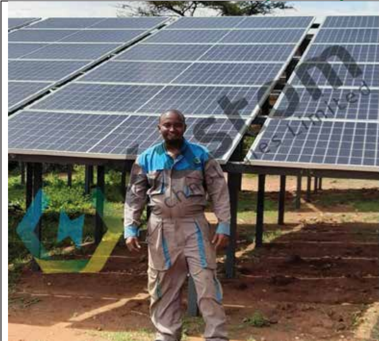
24 KWp Jinko | 24KW Jinko | 32 Kwh BYD Masai Mara Solar Offgrid System
