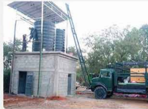
Borehole Solar Water Pumping
