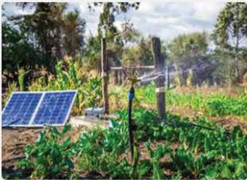
Agri-Business Solar Water Pumping
