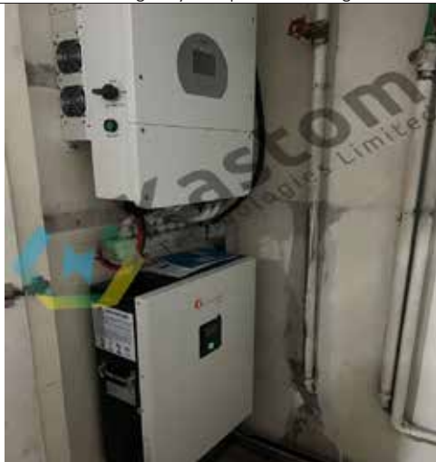
8KWp Jinko | 8KW Inverter Deye | 10 KWh Felicity Residential system - Loresho Nairobi, Kenya
