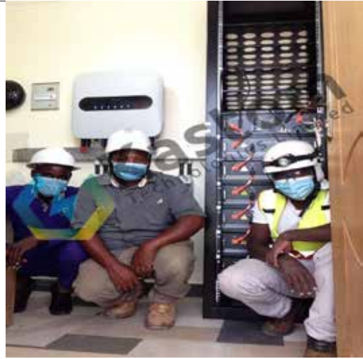
12 KWp Jinko | 10KW Sermatech | 40 Kwh Pylontech Residential ESS Ridgeways Nairobi
