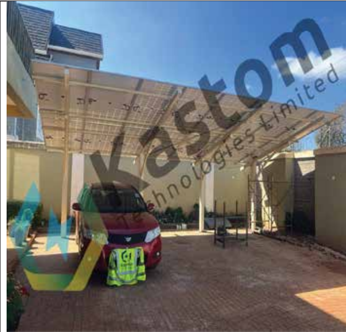
8 KWp Jinko | 8 Kw TBB Riiosun II | 10 KWh Eastman Lead Acid – Thika Greens Residential Carport
