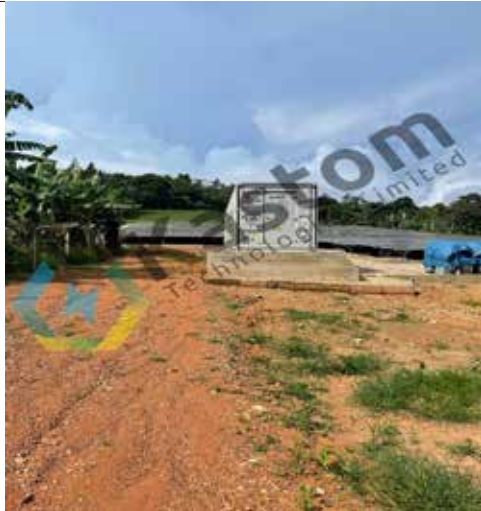
350 KWp Jinko | 300Kw -1.080 Mwh Jinko BESS Containerized Offgrid System | Busisi Island Uganda
